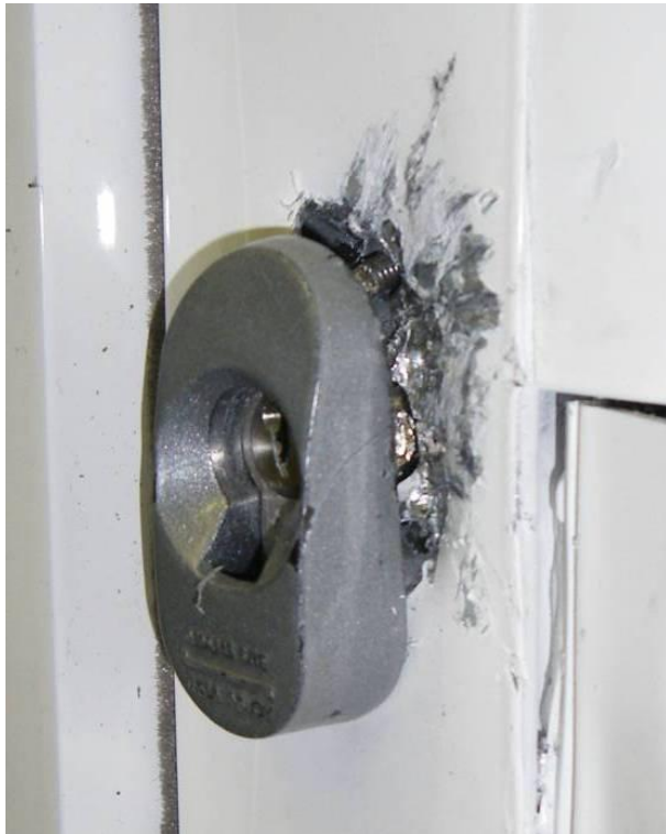
Figure 12 Damage sustained during attempts to lever off the lower escutcheon
