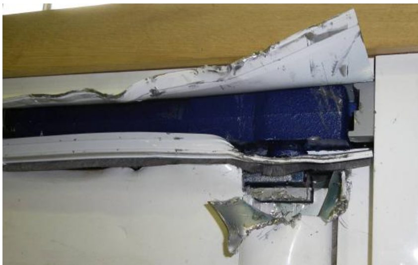
Figure 10 Damage to leaf sustained during attempt to isolate hinge, and damage to header sustained during attempts to overcome the door closer mechanism
