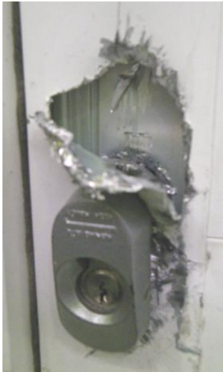
Figure 13 Damage sustained during attack test 18
