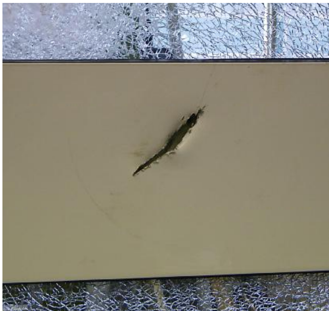
Figure 3 Cut created through outer layer of aluminium mid-rail profile
