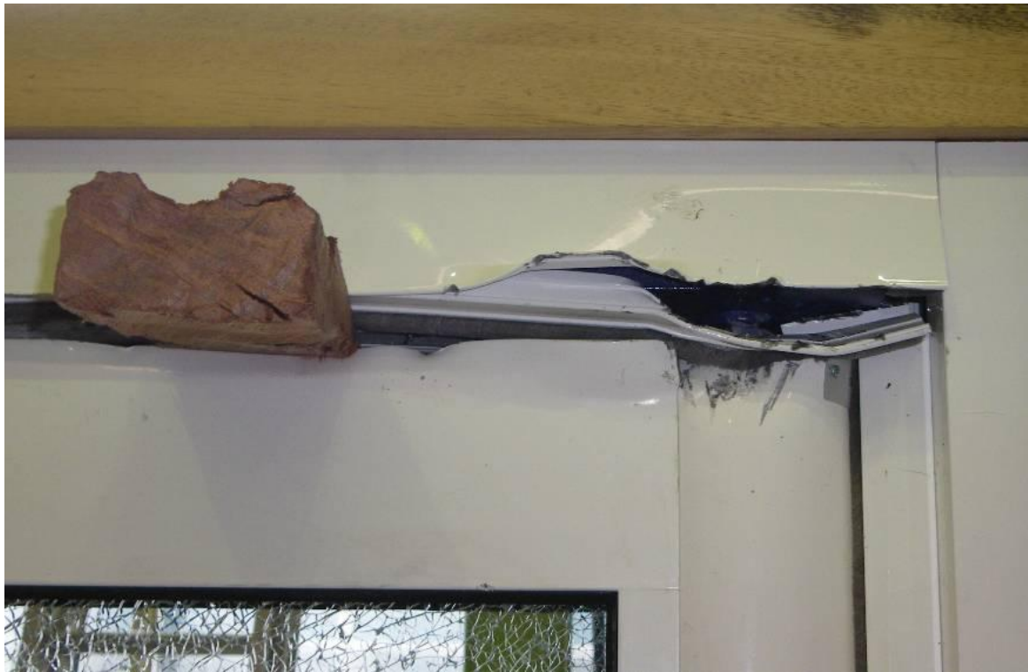
Figure 9 Damage as a result of attack test 10
